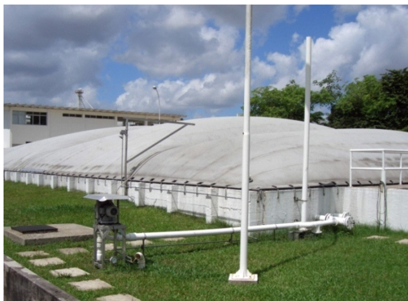
BIOLAK®GAS Liquid plant for a brewery of approx. 2 Mio. hl/a
